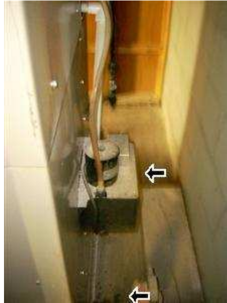
10.8 Picture 2 Leak at condensate pump
