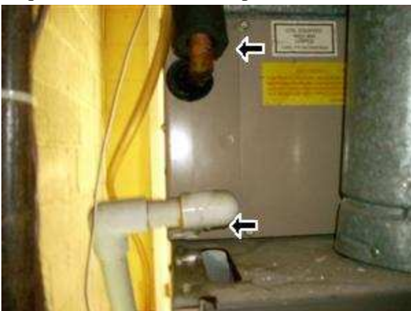
10.8 Picture 1 Condensation drip
