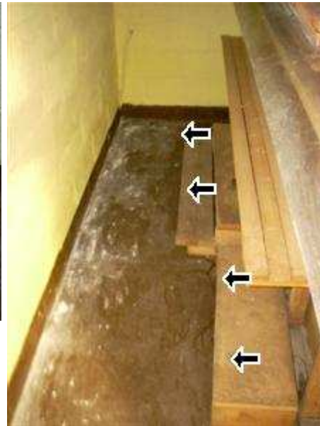
7.0 Picture 2 Moisture trails from back corner
