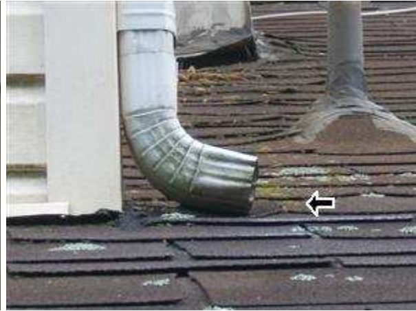
1.1 Picture 4 Note sag in sheathing
